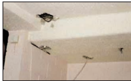
A ceiling coated with asbestos spray, which has been damaged by building work.
