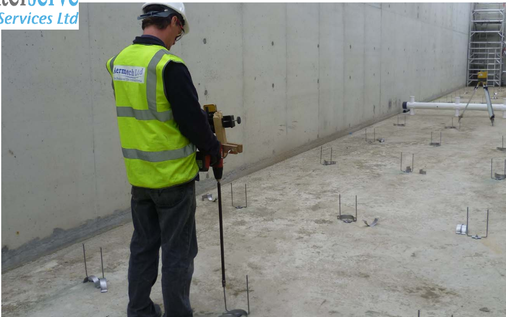
Using the right tools: long extension bit for the drill plus laser level attachment save hours of back breaking work!
