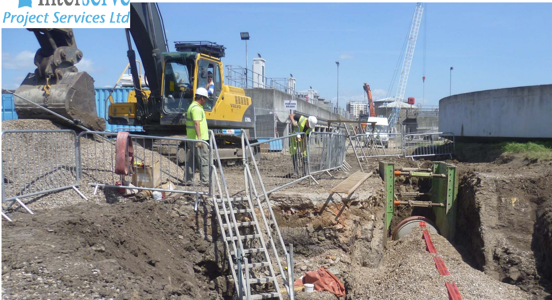
Open excavations are particularly hazardous. This gang has barriers to prevent falling and uses steps for all access/ egress.
