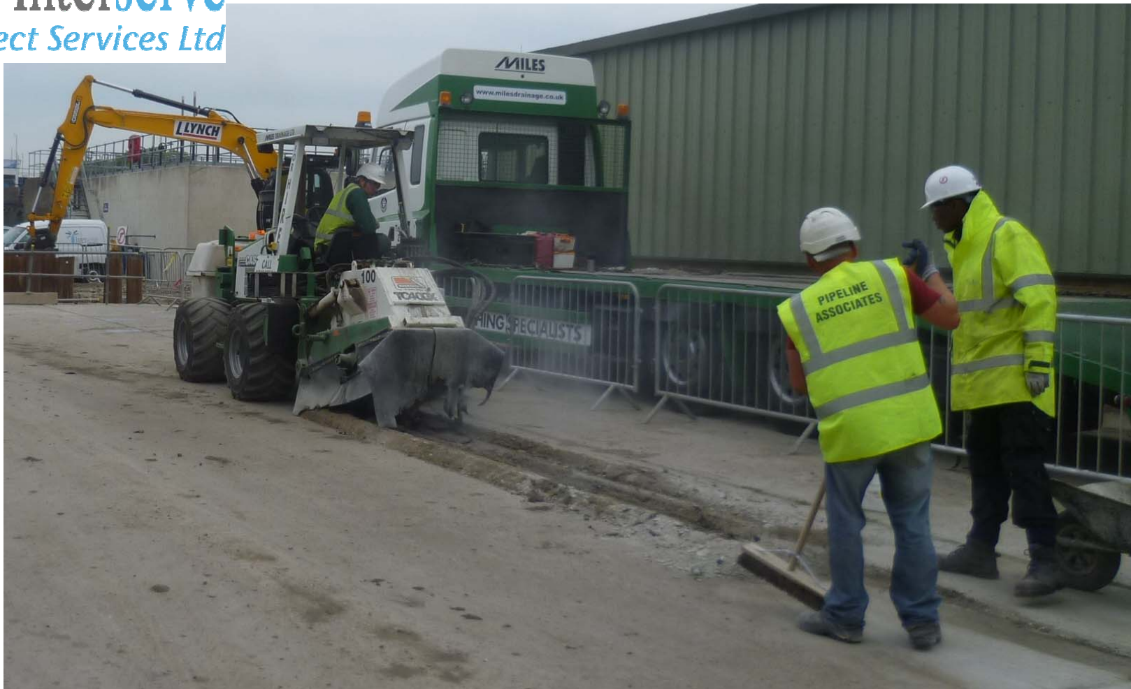
Integrated water sprinklers and curtains prevent dust, this cutter quickly grinds out the concrete without vibration or fuss.
