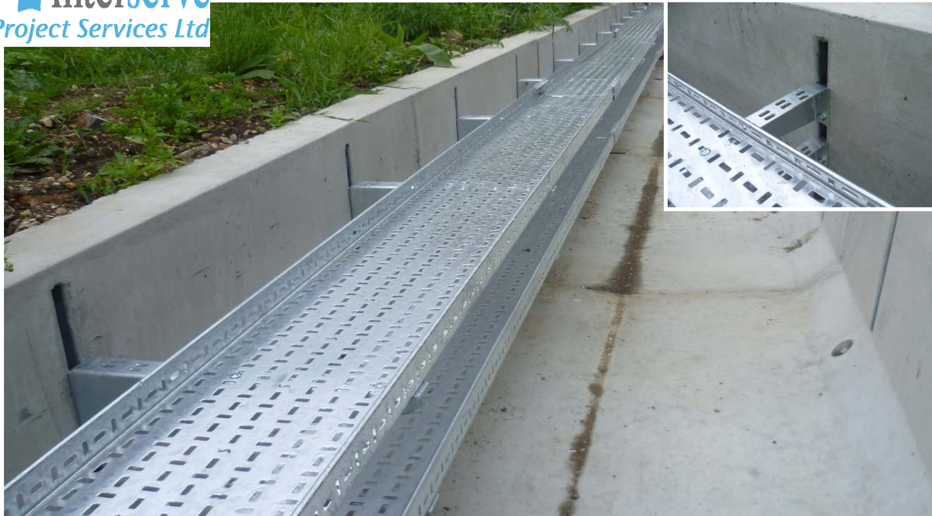
These trough units were cast with insets ready to receive the cable containment, avoiding drilling risks and saving time.
