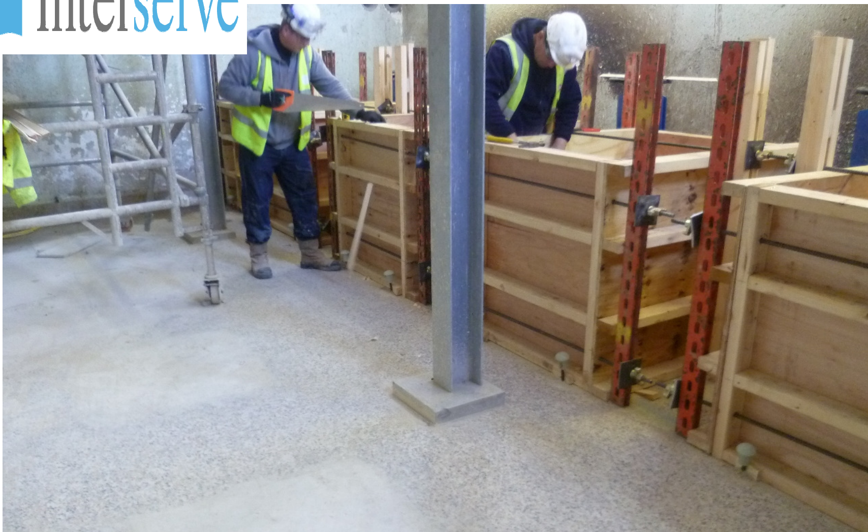
Working inside of existing pumping stations can be hazardous due to tight areas, access constraints and existing equipment.
