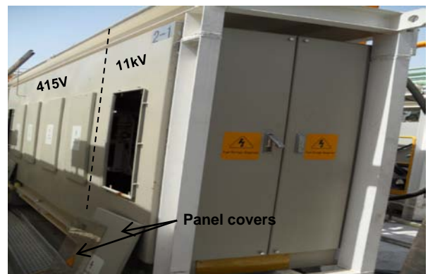
Figure 2. Switch gantry with 11 KV steel panel and polycarbonate screen removed.
