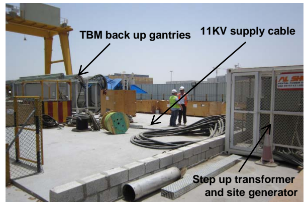
Figure 1. TBM back up gantries connected to step up transformer .
